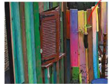
Distressed and weathered colourful cladding
